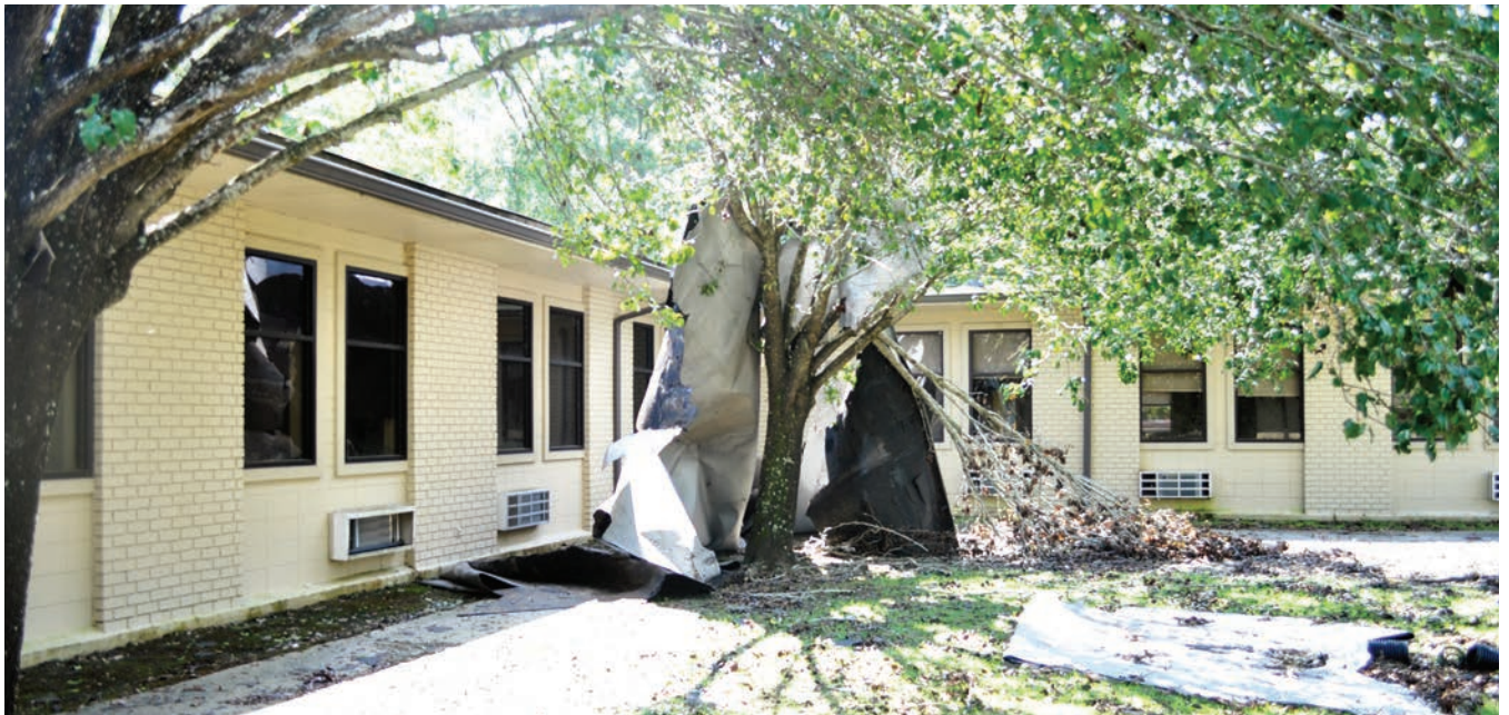
Ida's winds ripped a portion of the roof from the Covington building housing STHS's Express Care walk-in clinic as well as St. Tammany Pediatrics. Express Care has since returned to a portion of the building, while the pediatrics practice is operating out of the St. Tammany Physicians Network clinics in Mandeville and Madisonville. (Photo by Mike Scott / STHS)
