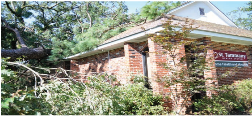
STHS's Home Health and Hospice building was destroyed by a tree during the storm. After working out of a conference room in Ida's immediate aftermath, the operation has since been temporarily relocated to the STHS Palliative Care office at 1010 S. Polk St. (Photo by Melissa Hodgson / STHS)
